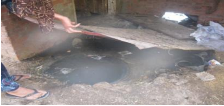
Broken Sewage System in Ezbet El-Nasr
